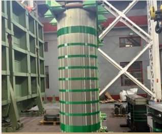
PRJ-01 330 kV EHV transformer core
